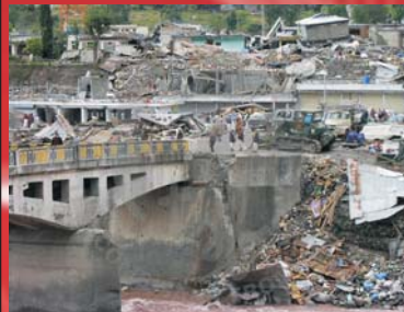
Balakot Bridge on Kunhar River in KPK Remained Intact But virtually Displaced
